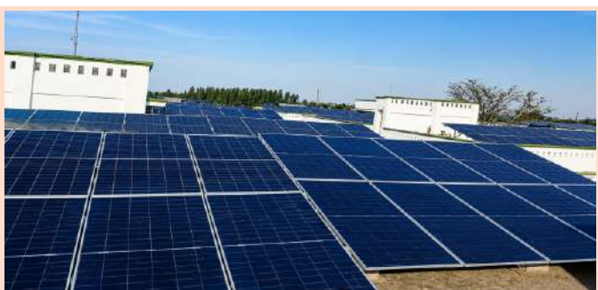
Capacity: 15MW Location: UPNEDA
