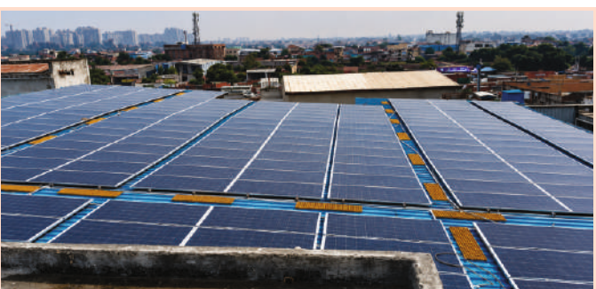
Capacity: 300kWp Location: Placero International Pvt. Ltd.(Sonipat)
