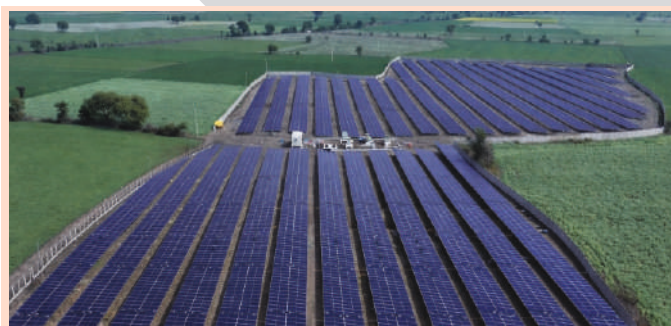
Capacity: 4.5MW Location: Ahab & Bhadora, MP Kusum Yojana
