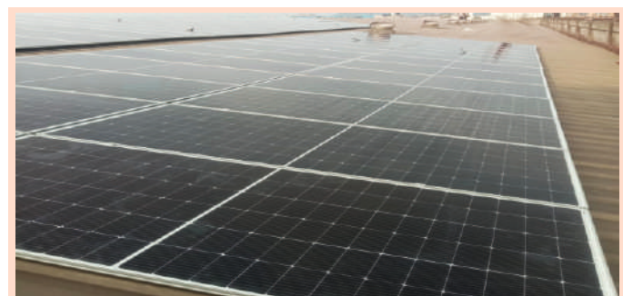
Capacity: 504 kWp Location: Awadh Rails, Haridwar
